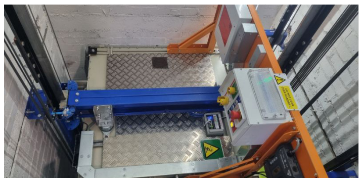
The car top of one of the modernised lifts
