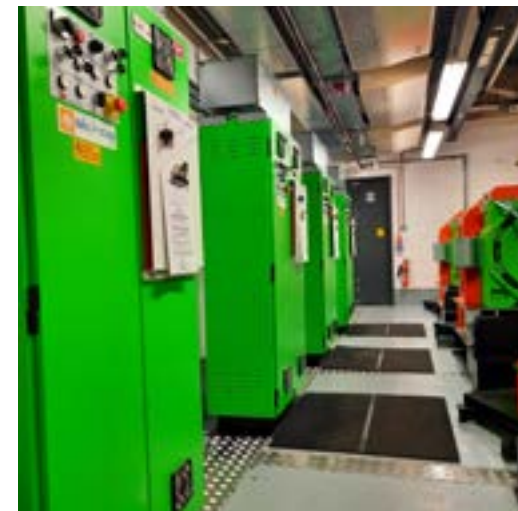
The upgraded lift control panels.
