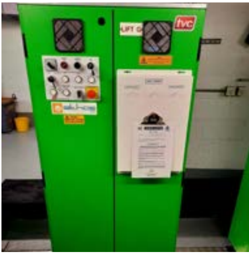
The upgraded lift control panel.
