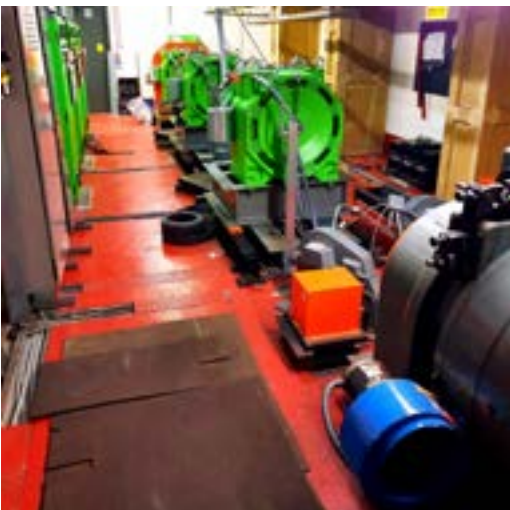
The modernised machine room.
