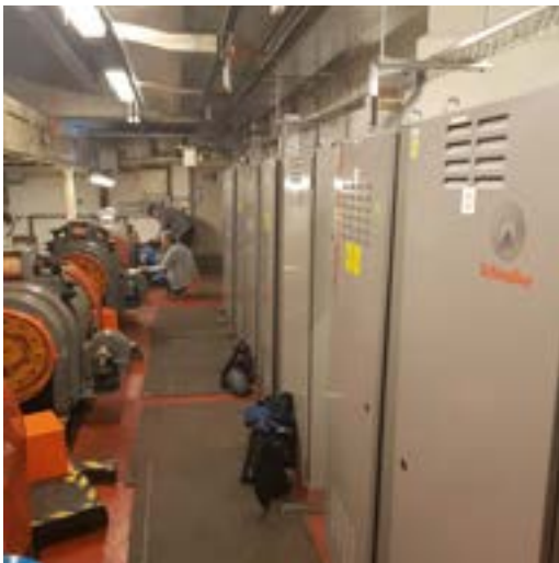
The old machines and control panels.
